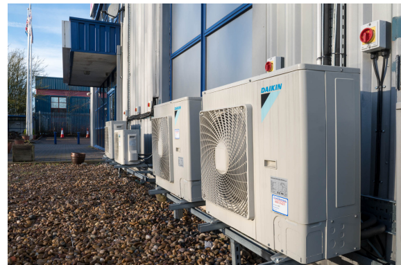
New energy efficiency units replaced old air conditioning
